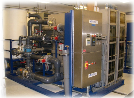
Membrane Filter in use at the Homestead Resort's Water Treatment Plant.
