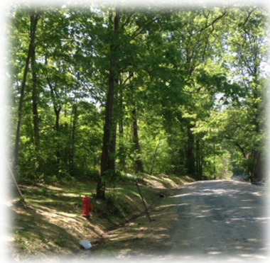
Above Photograph: Shows the 1 st Westridge hydrant installed on Muskrat Run Road. New ditch line and re-graded Muskrat Run Road to help protect newly installed line.
